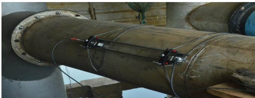
Fig. 3. Ultrasonic flow meter mounted on the delivery pipe of vertical submersible pump
